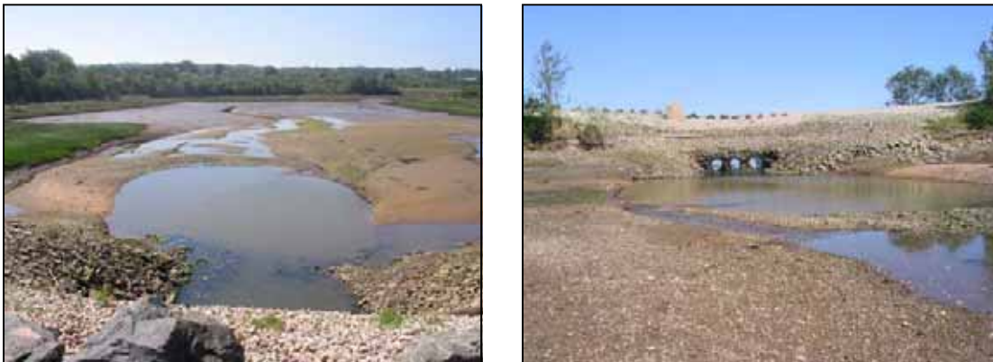
Figure 4: The landward view showing large scour pool directly above culverts (left), and a view of the culverts looking downstream (right)
