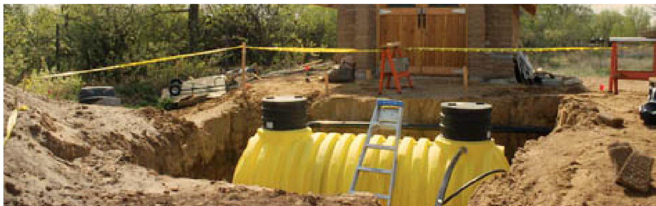
Installation of an underground cistern for a newly constructed house. Image taken from buildingwithawareness.com
