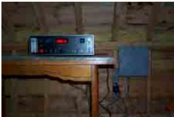
Inside - Monitor and Data Logger
