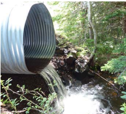
Perched Culvert in the Watershed
