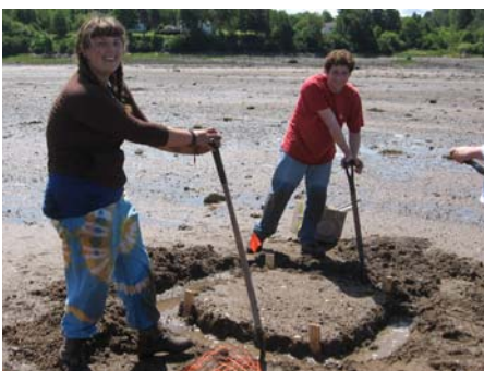
Staff members Megan Tardif-Woolgar and Jeffrey Glenen digging a trench to install snow fencing at Twin Cove Road.
