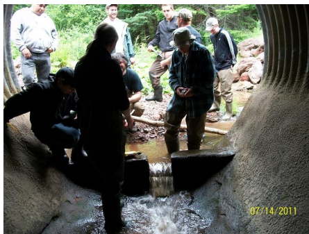
Participants assessing a culvert at the workshop in Truro. Photo taken by NSLC Adopt-A-Stream
