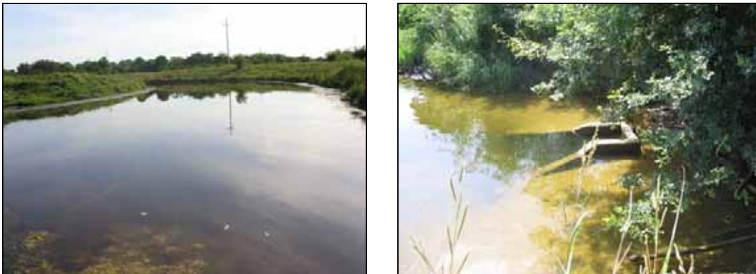
Figure 6: Landward side of dyke showing water pooling behind dyke (left) and photo of drainage structure on downstream side of dyke (right)
