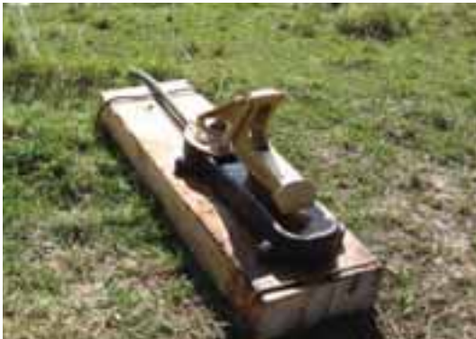
Figure 5- Nose pump installed on Bruce property.
