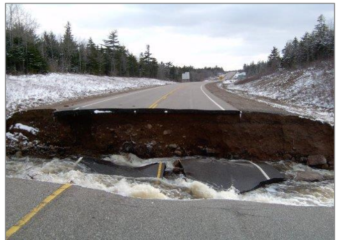
Photo location: Highway 101 Source: http://www.novaweather.net/Flood_2003/Flood_Hwy101b.jpg
