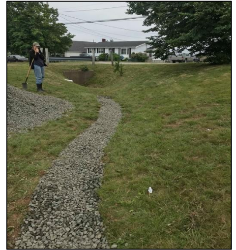
An infiltration trench located in Digby, Nova Scotia
