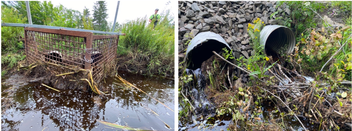
Figure 29. ALL017 inflow (left) and outflow (right) blocked with debris.
