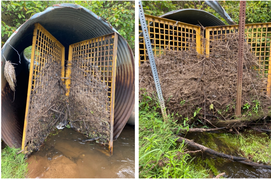
Figure 34. TRO010 inflow before the debris removal.
