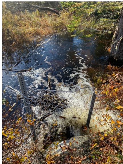
Figure 19. Culvert grate blocked with debris.
