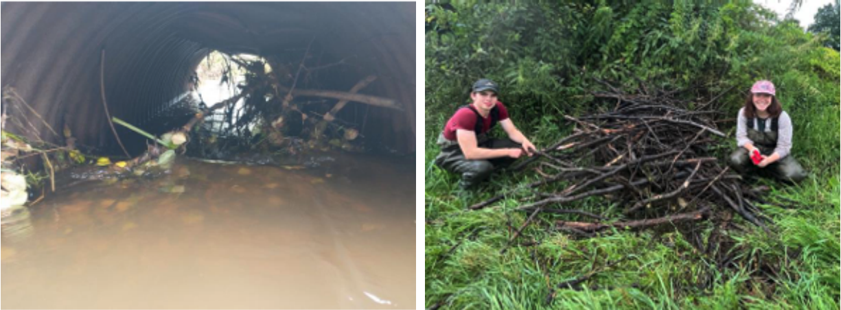
Figure 38. BWB003 before (left) the debris removal and JWA staff (right) with the debris removed from the site.
