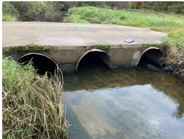
Figure 39. BWB003 after the debris removal.
