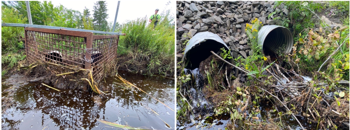
Figure 8. ALL017 inflow (left) and outflow (right) blocked with debris.
