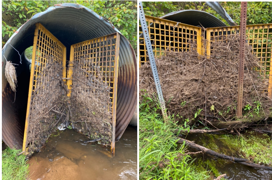
Figure 13. TRO010 inflow before the debris removal.
